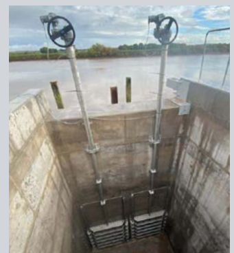
Penstocks with operating gears
