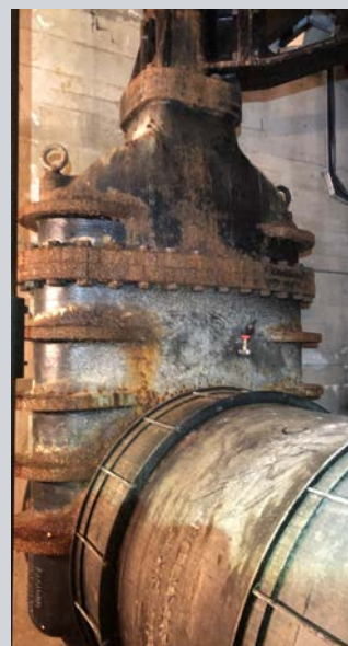
The original valve
