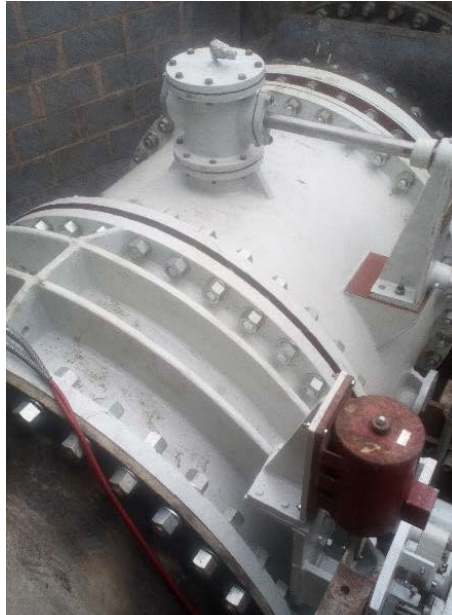
Refurbished valve and operating arrangement
