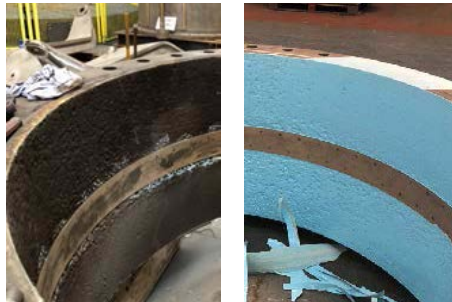
Internal bore of valve body and seating face - before and after
