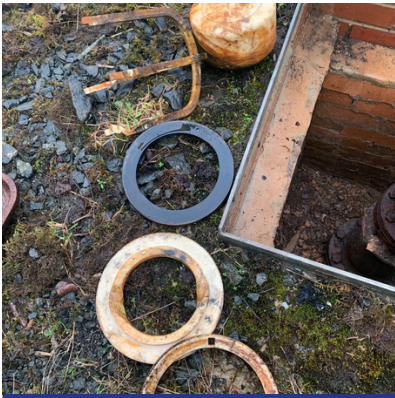
The original air valve
